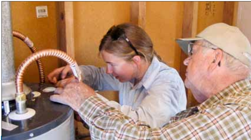
Miriam Regier with MVS and Walter Good with SOOP fix a water heater as part of a home repair ministry started by SOOPers and Shalom Mennonite Fellowship in Tucson, Ariz.
